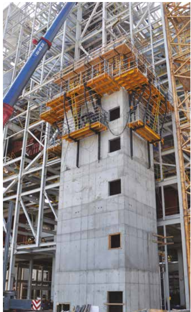
The ATR system works without crane and under adverse weather conditions. Moreover, its large platforms and handrails ensure workers' safety.
