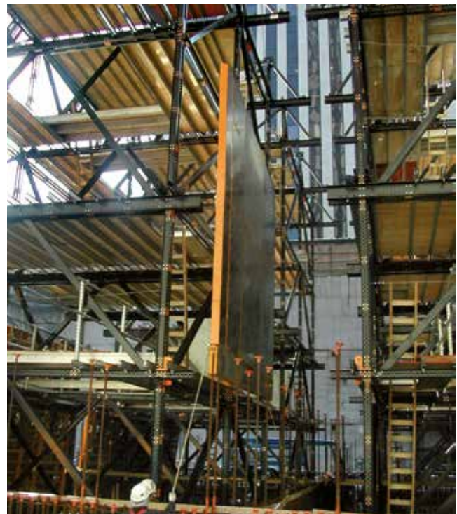
The self-climbing technique consists in a hydraulic system that enables automatic lifting by successive movements of structure and masts.
