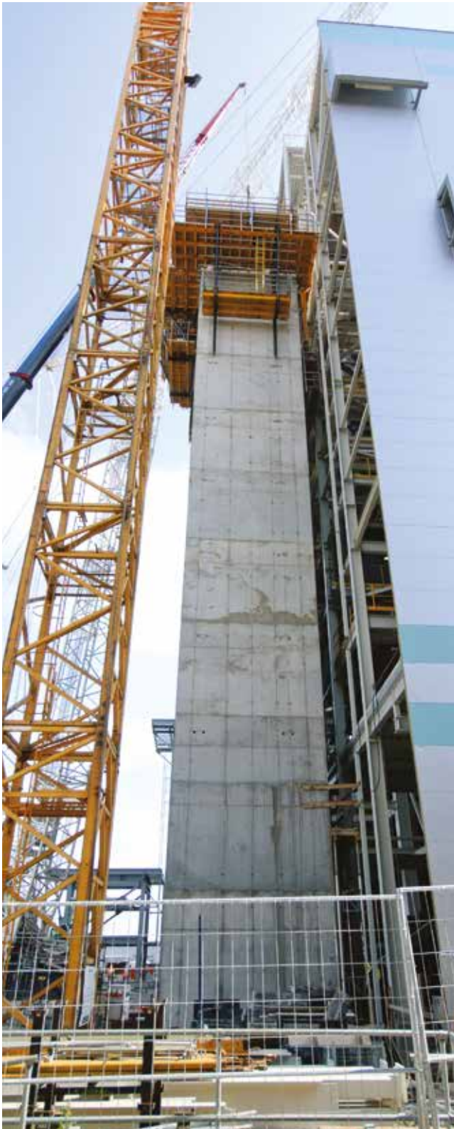
The vertical communication of the building was solved with the construction of two lift shafts.
