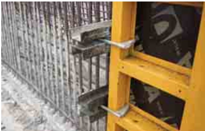
▲ Fixing the Waler to the Panel using Bulkhead Hooks tied to the profile
