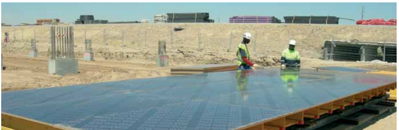
▲ Assembly of Table VR horizontal formwork with phenolic plywood and VM-20 timber beams
